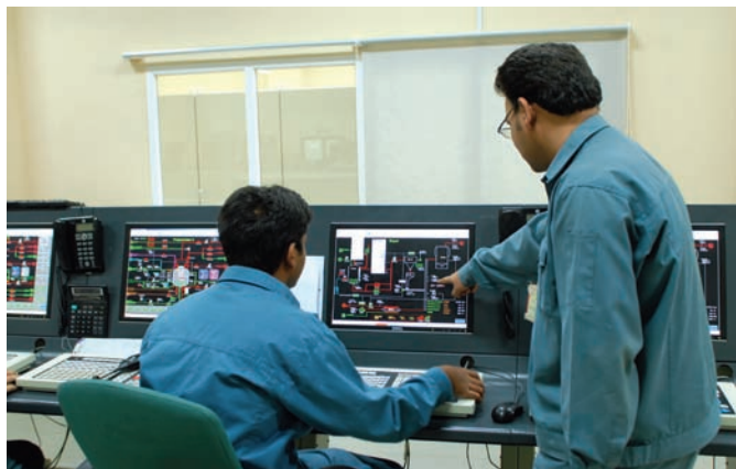
Central Control Room (CCR) at Plant Site
